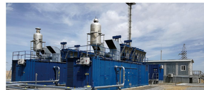
● Kazakhstan Oil Co.High-Power Units
